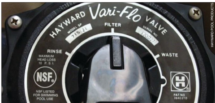
Multipurpose multivalve: This view of a sand filter multiport valve shows its various modes or functions, from filtering to backwashing to waste.
